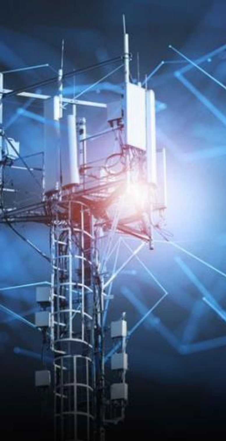
Telekom - LTE 4G - 5G
